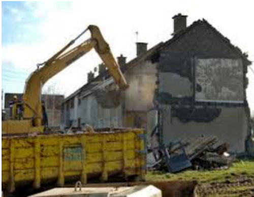
Addressing the poor quality of the housing stock, demolition work has begun
