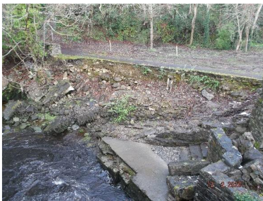
Swan Park has suffered recent flood damage. Locals and visitors look forward to the reopening of this important amenity.
